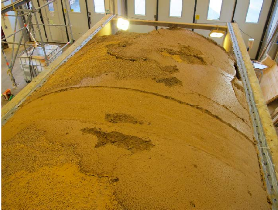
Figure 5-9. Photo showing the pellet ceiling after having removed the steel roof in Test 5.
